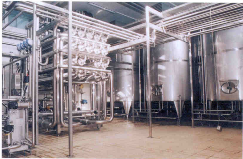
Crystallization tanks for permeate and/or whey concentrate.
