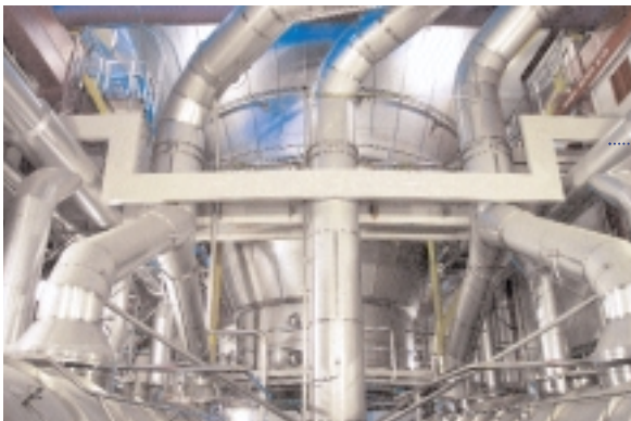
Multi-stage drying plant with integrated fluid bed. Three Vibro-Fluidizers® for products after drying/conditioning are placed below – only two are visible in the photo.
