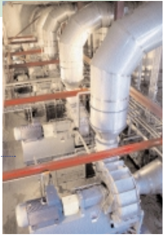
6 MVR compressors for 3 falling film evaporator plants.
