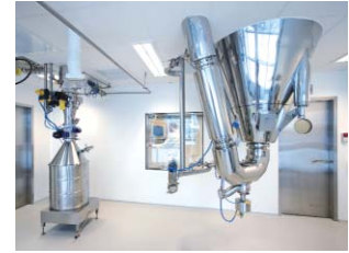
PSD-4 chamber cone in cleanroom
