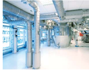
PSD-4 chamber and HVAC ducts
