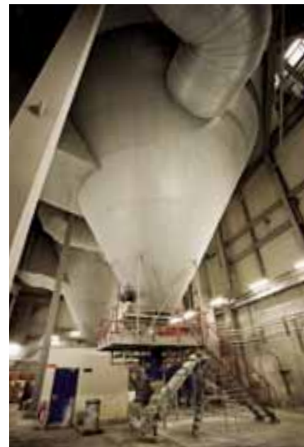
Bottom of SDA with flue gas inlet and outlet duct and product discharge.
