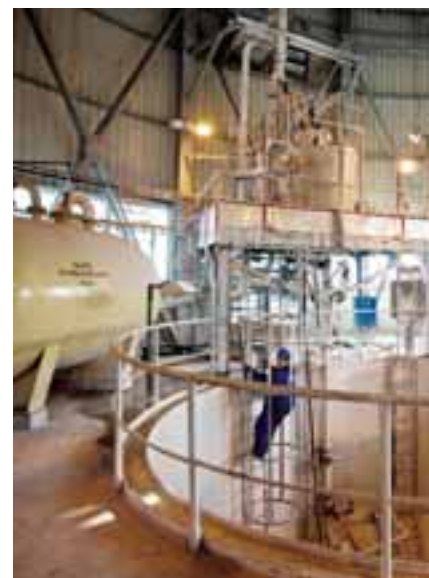
Absorber penthouse with absorbent supply arrangement and spare rotary atomizer.
