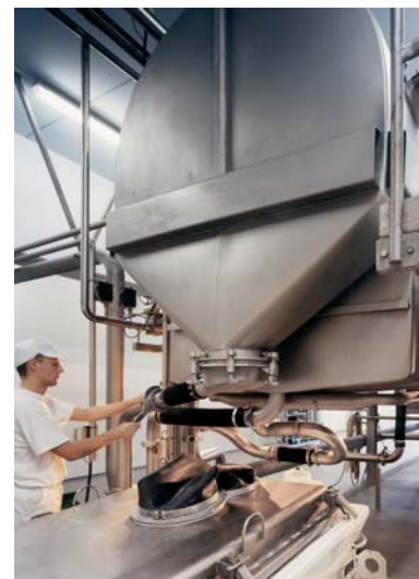
Preparing the VIBRO-FLUIDIZER® for CIP cleaning by placing a tunnel which returns the cleaning liquid to the CIP kitchen
