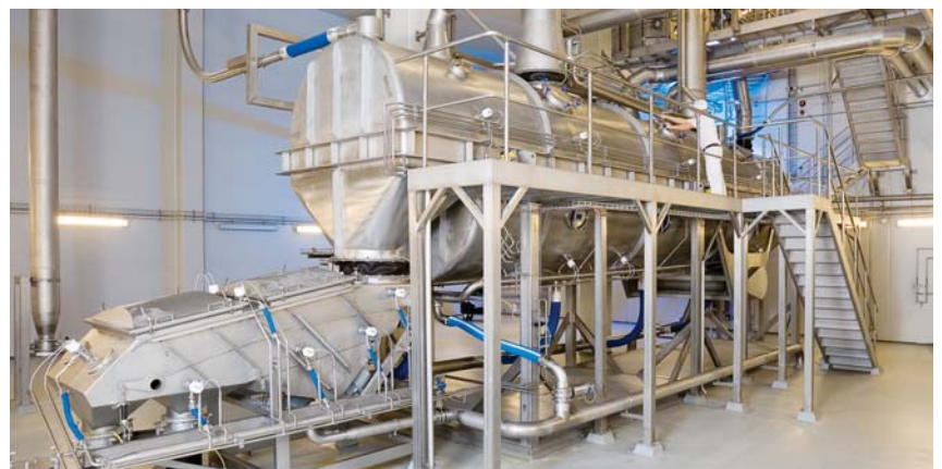
VIBRO-FLUIDIZER® and sieve with side-mounted CIP nozzles
