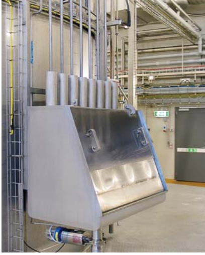
High pressure atomizer nozzles ready for CIP cleaning. All nozzles lances and nozzle heads are placed in a special stand for cleaning
