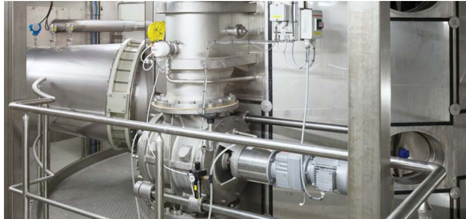
CIP nozzles installed to clean the integrated fluid bed and the spray dryer
