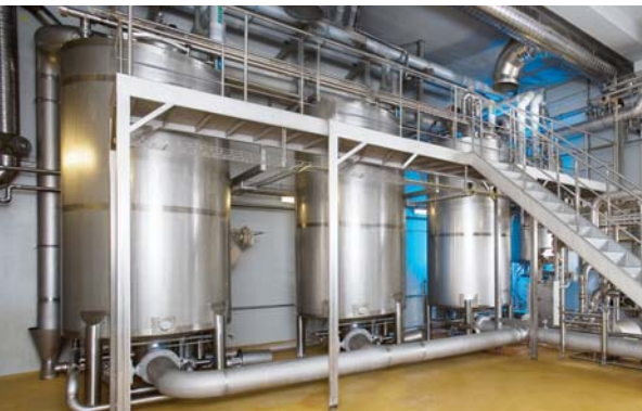
CIP kitchen with four tanks
