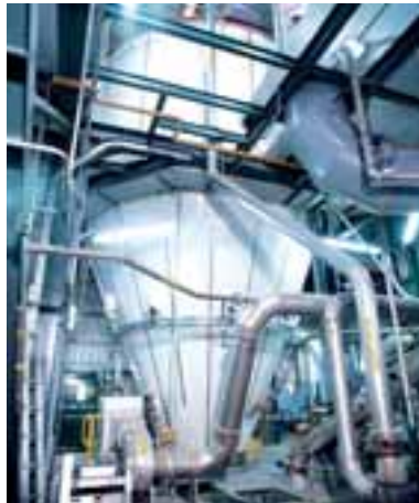
This spray drying plant in a semi-closed configuration includes incineration of exhaust bleed
