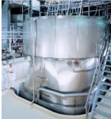
Top of drying chamber showing air disperser
