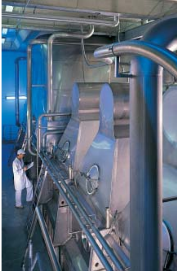
Final drying sections with venturi design for air-flow
