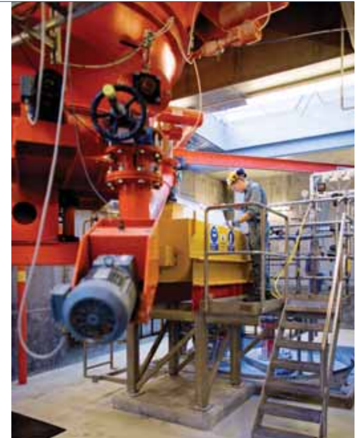
Lime slaking system at a Danish waste incinerator.
