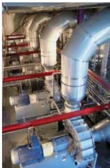
Falling film evaporator with mechanical vapour recompression (MVR)
